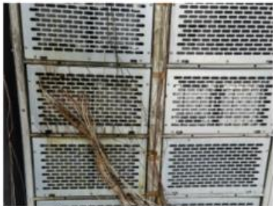
Figure 28a. Photo of thermal runaway location.
